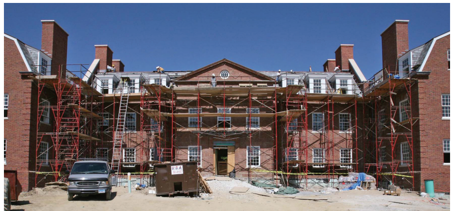
Evergreen slate roofing being installed at a New England boarding school applying for LEED certification.
